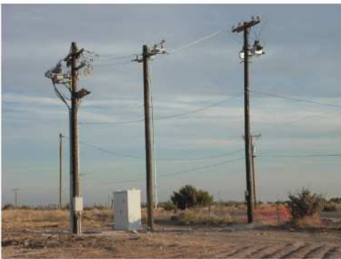
Point of Common Coupling Equipment
